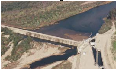
Vern Freeman Diversion Dam on the Santa Clara River & its Impossible Fish Ladder
